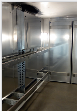
Technical service duct fitted vertically for easy maintenance and cleaning
