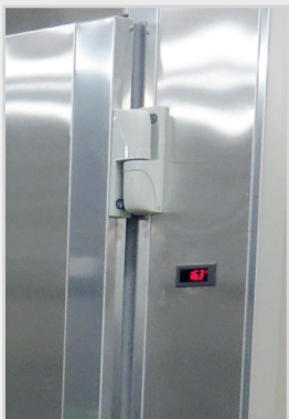
Temperature display on the exit side of the trolleys
